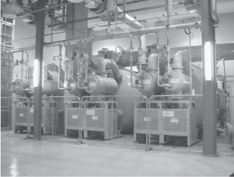
Haymarket substation (Australia)
